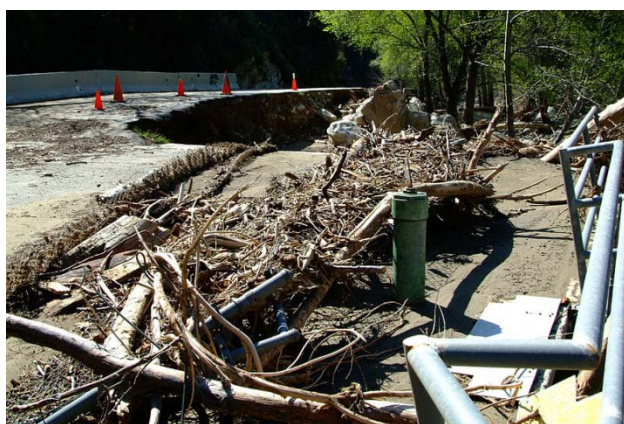
Figure 50: Road damage after flooding, wildfire or landslides are just some of the risks from climate change to transportation infrastructure. (Photo: FEMA)
