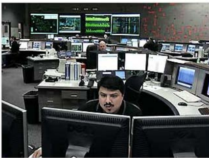
Aug. 3: Andrew Mann, a grid resource coordinator at the California Independent System Operator, monitors power use at the ISO control room in Folsom. AP
