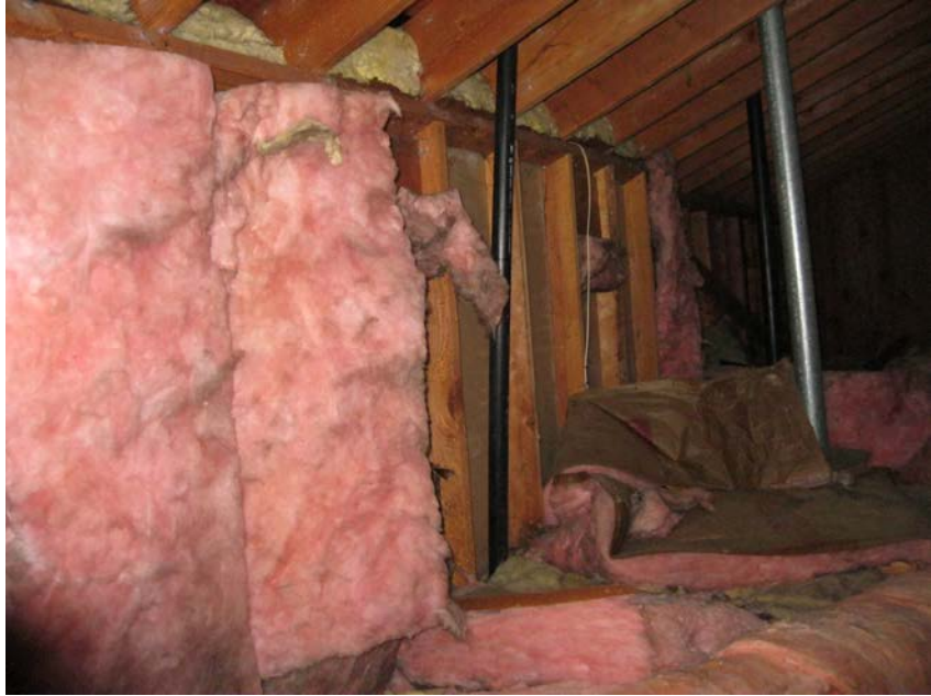
Improper knee wall insulation
