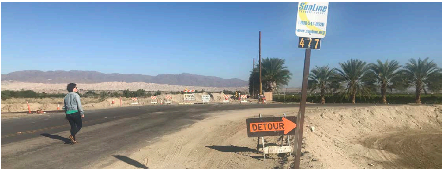
The bridge at Ave 70 and Cleveland St in North Shore, 1 of 2 entry points into the neighborhood, while under repairs
